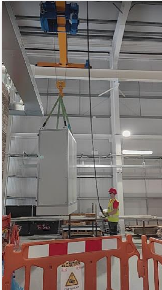
Example of use of gantry crane by certified person, certified and tagged equipment.
