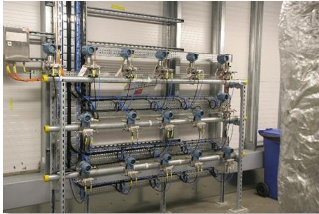
Example of an on-site FOK
